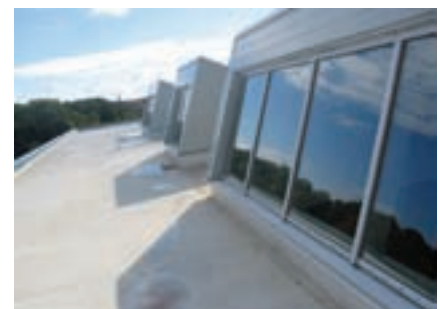
Skylights atop the Earth Rangers Centre are a testament to their commitment to green friendly
